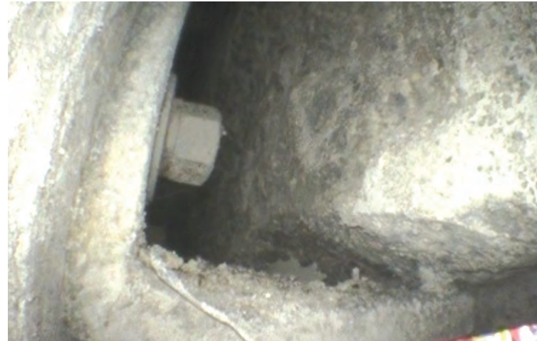
Irregular bearing surface on bottom side of panel not fully in contact with relieving angle
