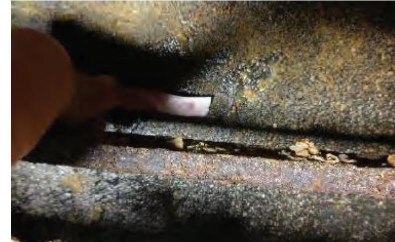
Concrete back-up wall: Water saturation
