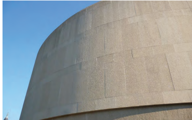
Overall photo of exterior precast concrete panel cladding on outer ring: Note the interchanging rows of large and small panels and staggered vertical joints between rows.
