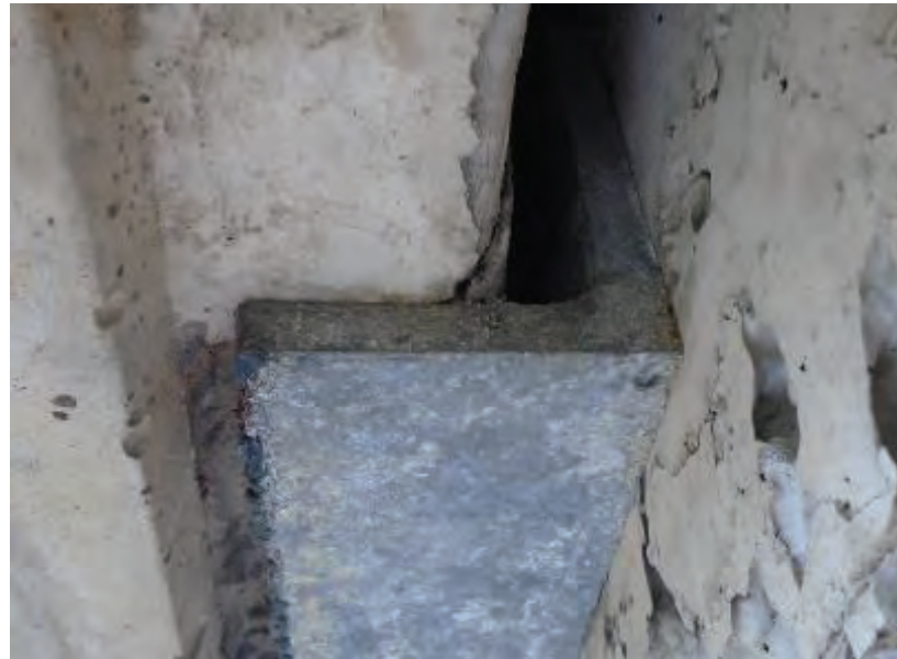
CRACKED CONCRETE AT THE RELIEVING ANGLE
