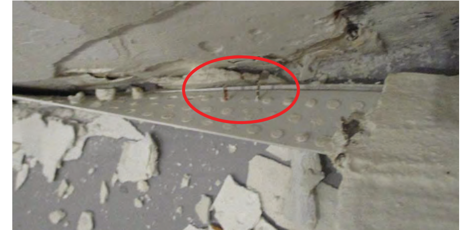
Delamination and flaking plaster at the base of the wall finishes at the second level gallery due to the moisture inside the wall assembly.
