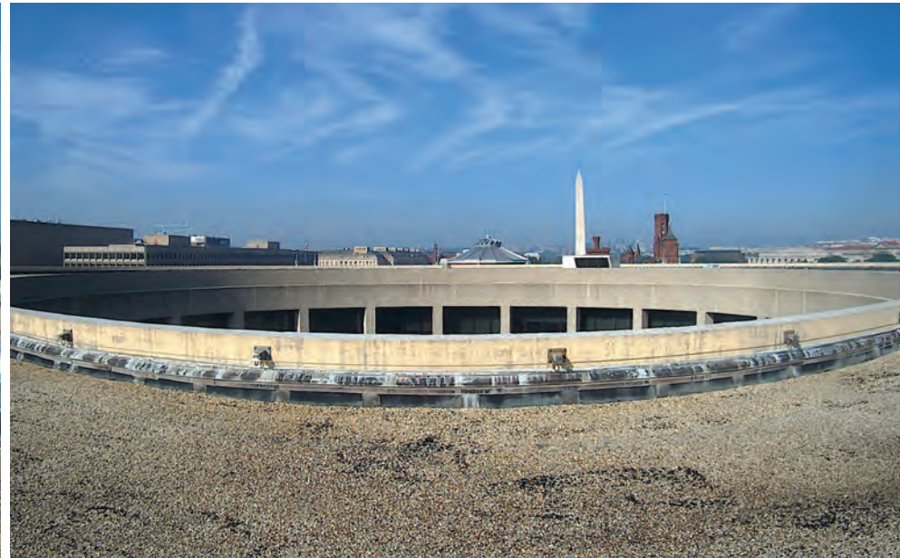
Roof assembly and fall arrest system
