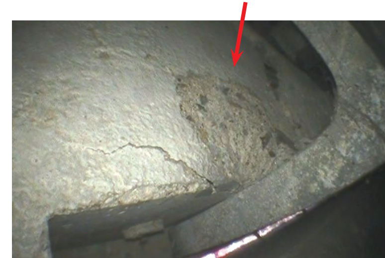
Backside of the concrete panel is cracked adjacent to the bearing surface on the relieving angle
