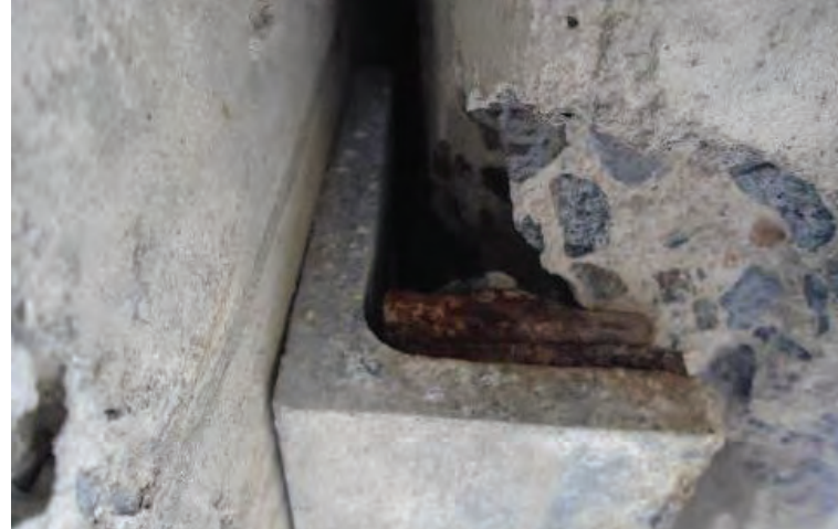
Relieving angle: Corrosion, spalling, and uneven panel bearing
