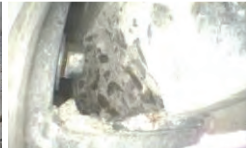
Concrete spalling adjacent to relieving angle bearing surface
