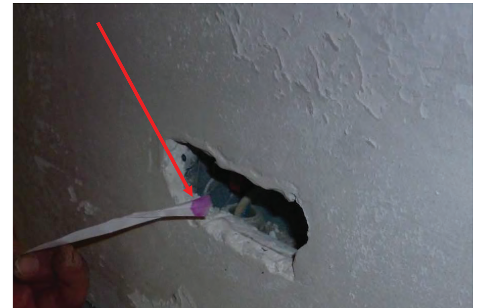
Water finding test paper indicates the presence of moisture on the interior face of the backup wall behind an electrical outlet.
