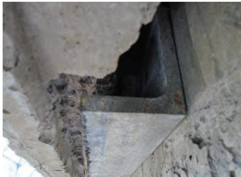
SPALLED CONCRETE AT THE RELIEVING ANGLE
