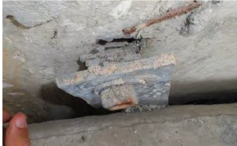
Strap anchor: Shims filling gap and strap bent
