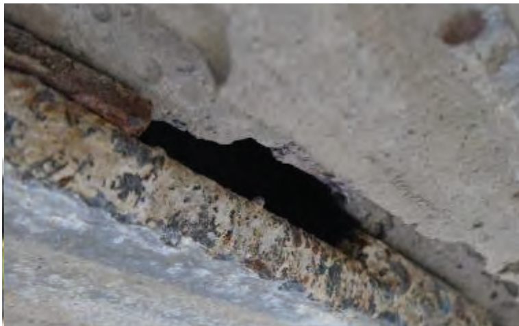
View of the bottom edge of a large panel: The back edge of the recessed pocket has spalled off the panel and does not engage the relieving angle bar
