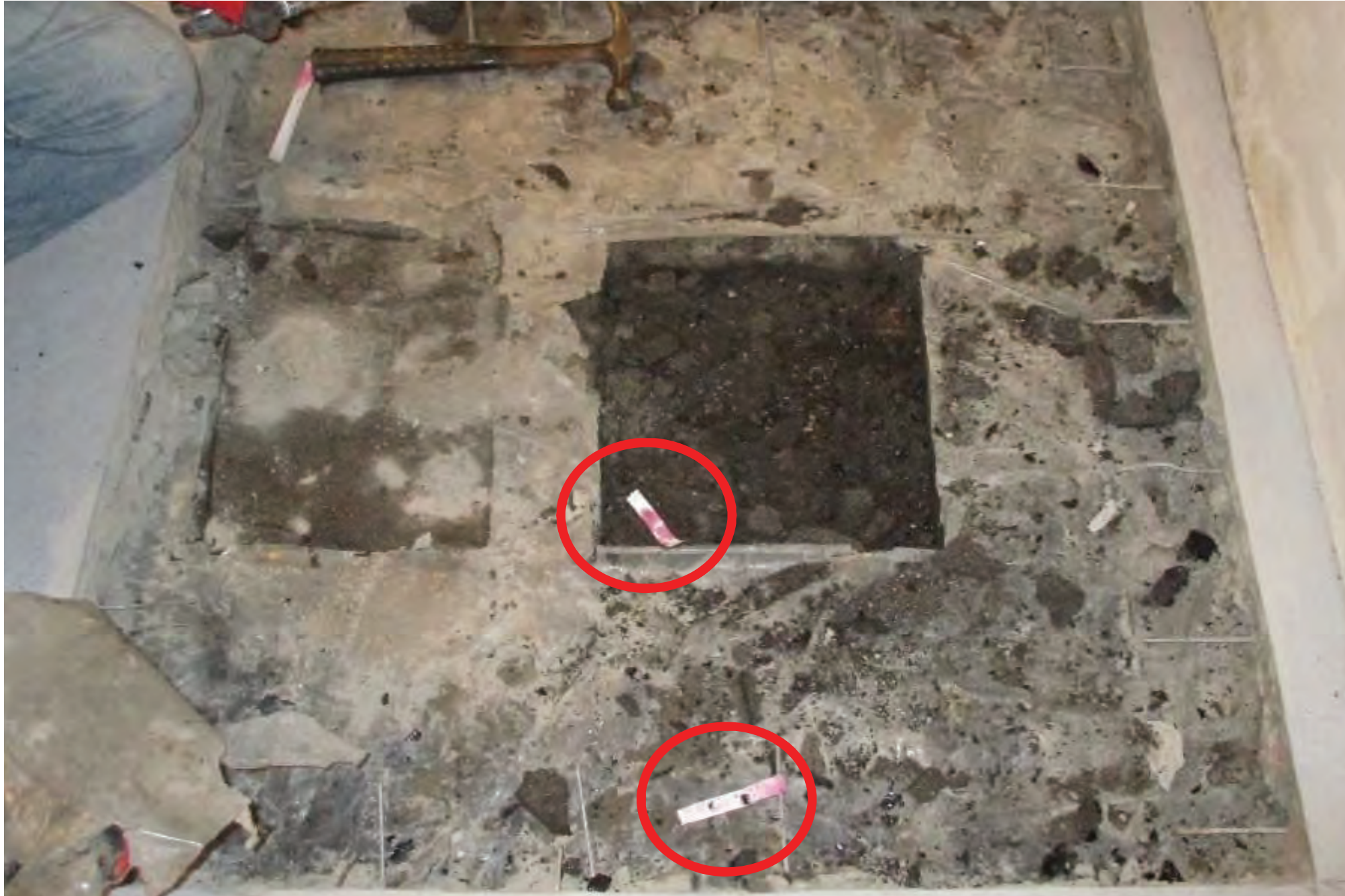
Pink discoloration of water finding test paper indicates moisture in the glass foam insulation of the Second Level Slab Assembly.
